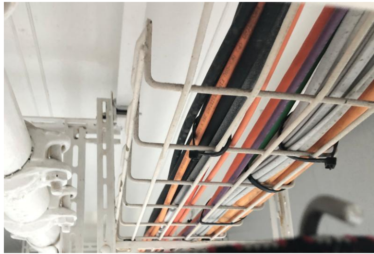
Figure 1: Cables on Emerald Princess (Photo by Norbert Doerry)
